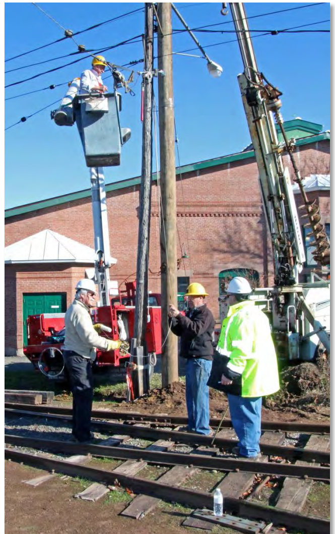
Bill Stolba (in bucket) & (L to R) John Arel, John (Kurlicie) Kurlick and Al Goff work on replacing a pole in Kelly Yard.
