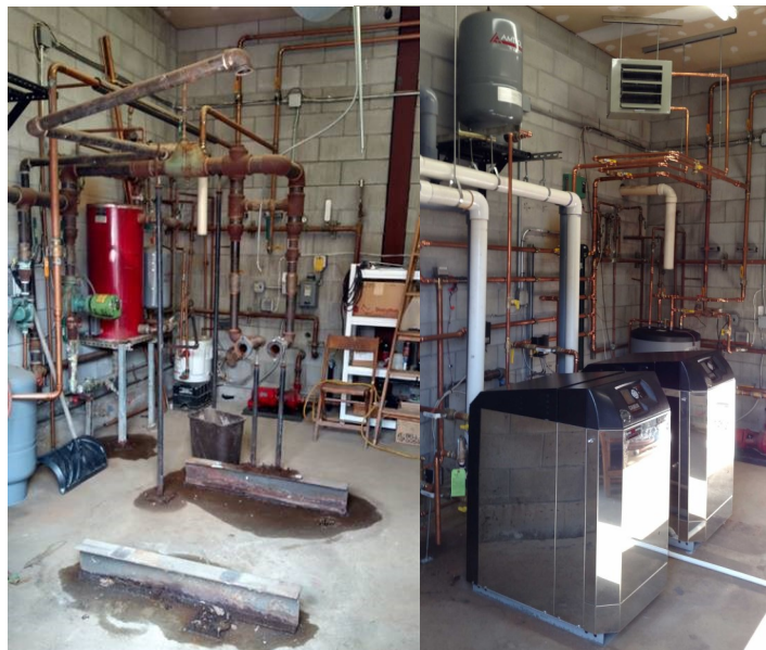
New Boiler installation for the Visitor Center; in progress (left) and completed (right)
