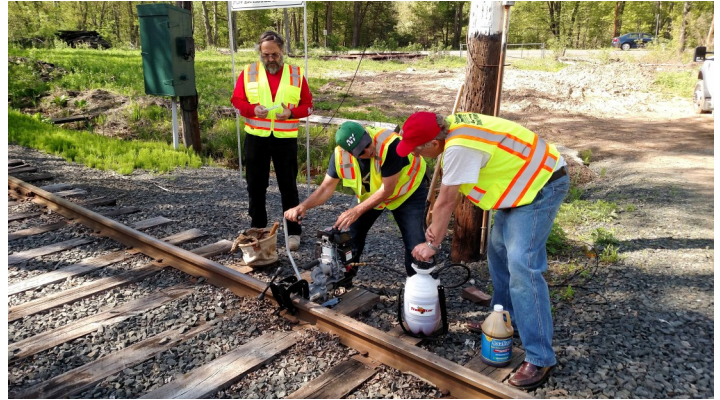
Signal Bonding at Powerhouse Crossing
